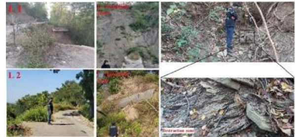
Fig. 11. The Landslide Area.
